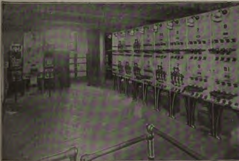
SWITCH ROOM OF NIAGARA FALLS POWER HOUSE.
